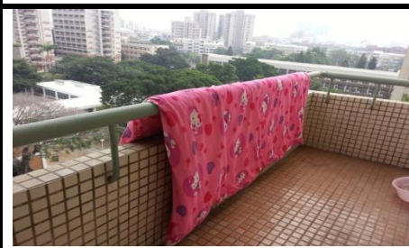
陽台 (×) Balcony personal belongings in the balcony
